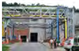
Energetski most in ukrep Ravne II
